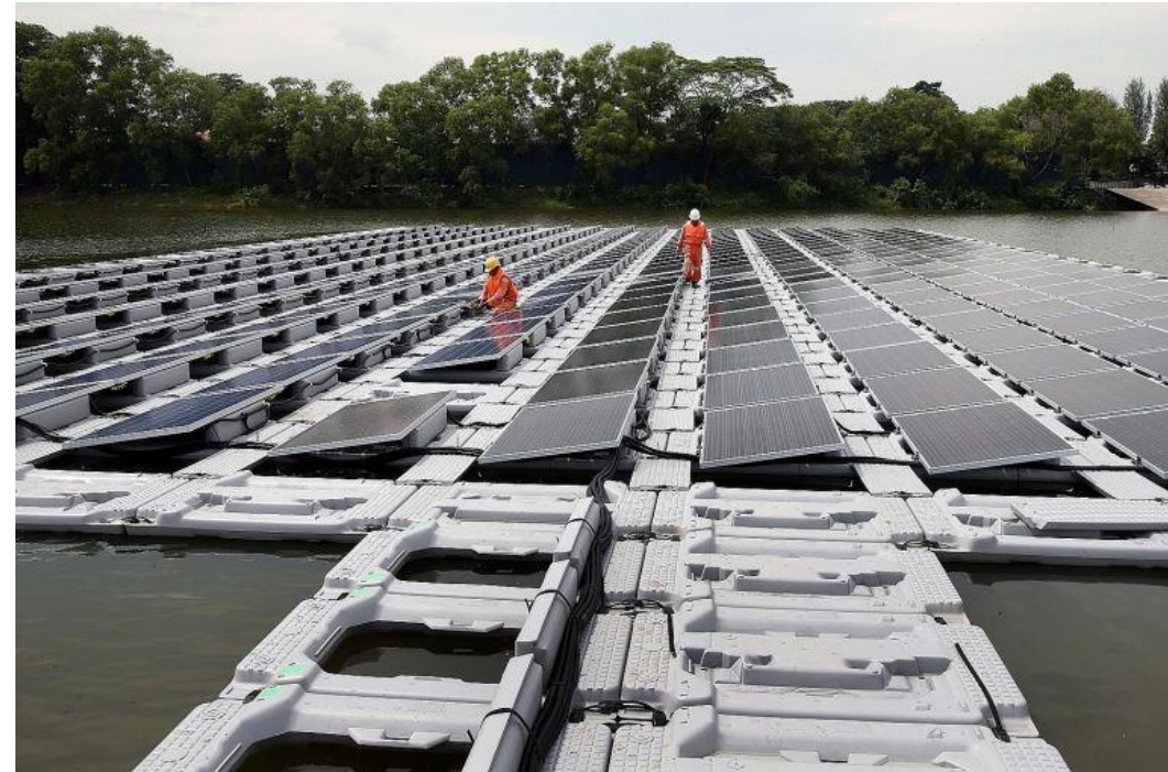
Floating photovoltaic cells test-bed at Tengeh Reservoir
